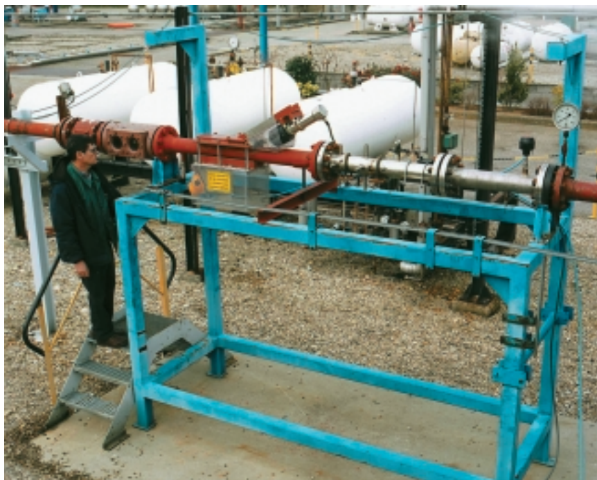
Figure 1b View of the reference venturi meter spool piece with the gamma densitometer and the flow visualisation window.
